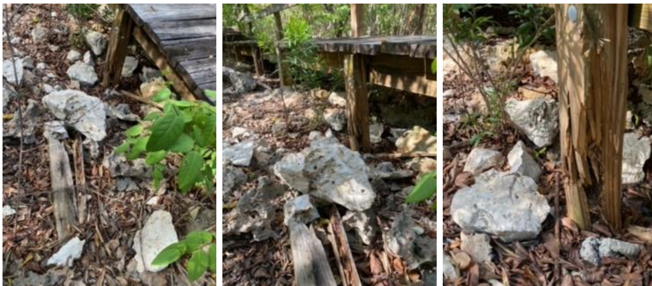
Figures 4-6: DoE site visit photos showing fly rock from the West End Quarry on the Salt Water Pond Trail and damage to the Salt Water Pond Trail boardwalk. (Source: DoE, taken: 30 March 2023)
