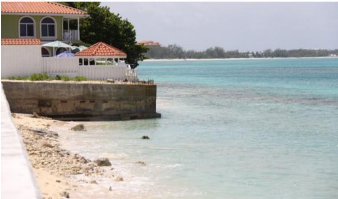
Picture 7: The site in July 2012 shows there was no beach directly in front of the property. The top of the seawall does not appear to be level when compared with previous photos, and the seawall footings are exposed, indicating there may be impacts to the structural integrity of the wall only two years after construction, and prior to the construction of any structures.
