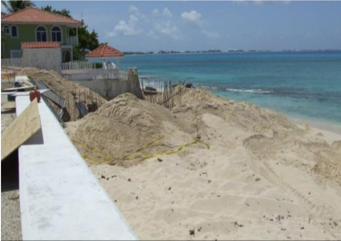
Picture 2: Construction of the existing seawall commenced in 2010. There are visible excavator tracks on the beach and in the water, which is a Marine Protected Area.
