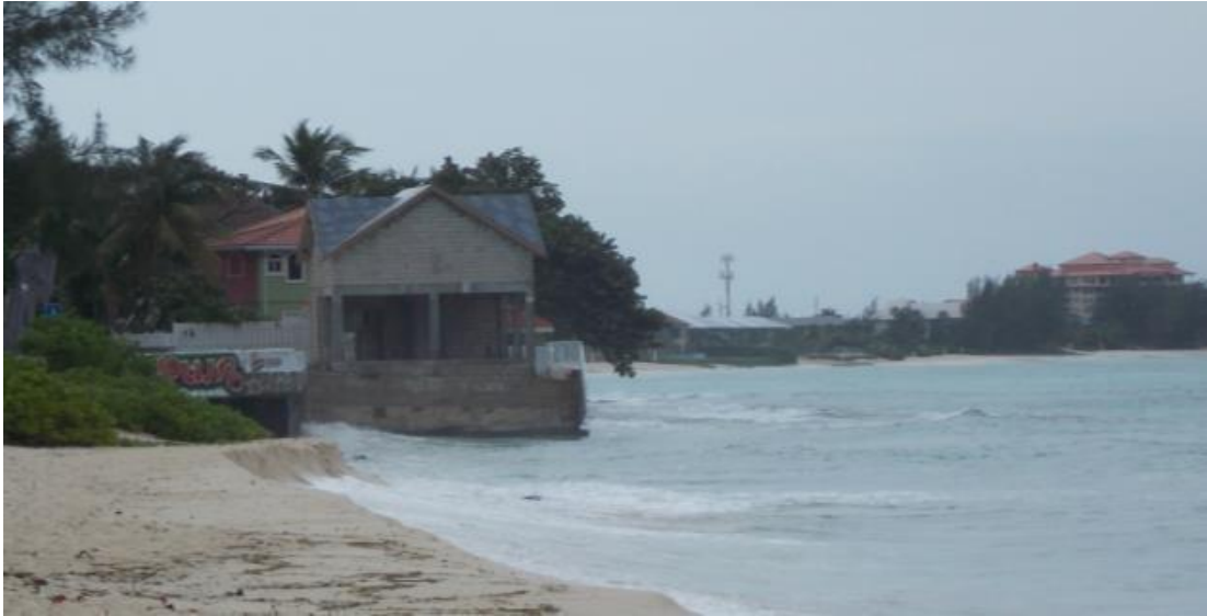
Picture 8: This photo of the site from September 2013 shows that gazebo is under construction and there is no beach on either the west or the north of the site. There are cresting waves along these two sides of the seawall. The seawall appears to be undermined or the footings are exposed.
