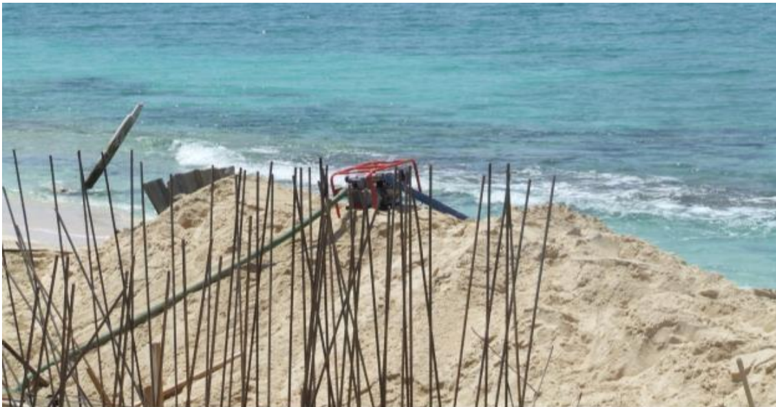
Picture 3: A pump can be seen with the outlet from the excavation into the Marine Reserve. The works had been stopped at this point.
