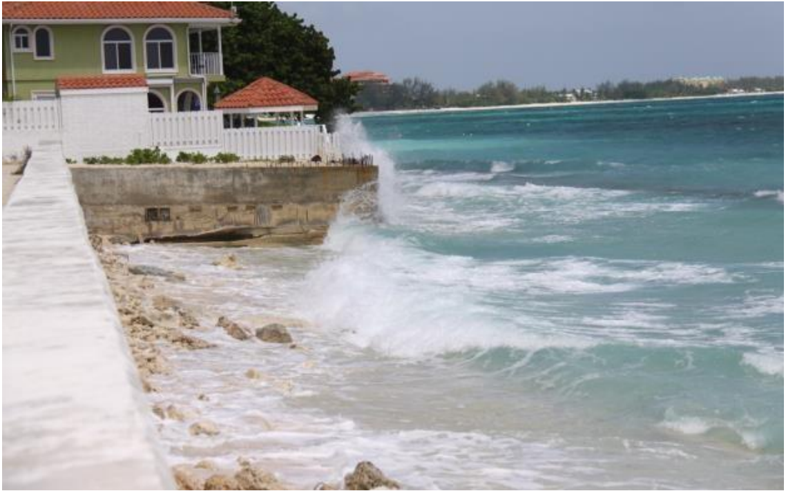
Picture 6: During a period of inclement weather in June 2012, breaking waves can be seen crashing against the seawall and cresting waves can be seen just offshore. The proposed house includes glass railings at the top of the seawall, where the waves can be seen breaking. The living room of the proposed house is just over 5 feet from where the whitewash can be seen.
