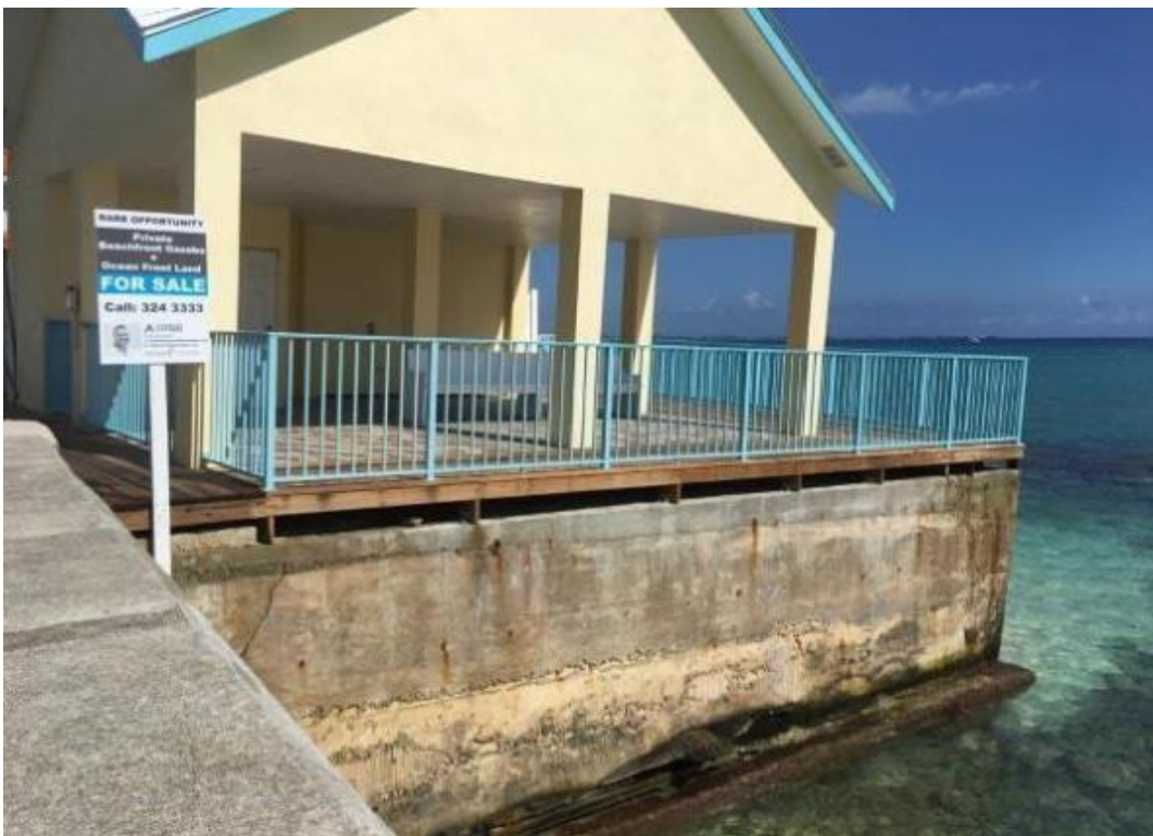
Picture 9: The site in August 2019 (photo from Cayman New Services) shows visible undercutting of the seawall as well as no beach to the south and west of the site.
